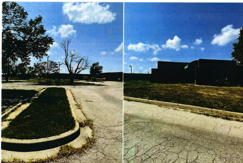
Figure 2 – Site Photos As Currently Existing Showing Degradation of Site
